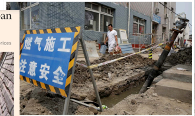
pipeline construction on the outskirts of Beijing. There is a demand-supply gap for gas after coal st...
