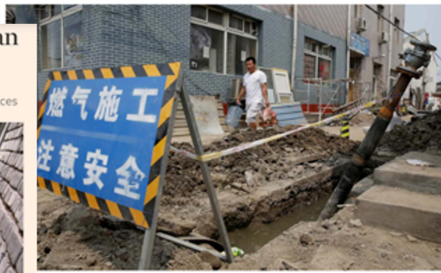
pipeline construction on the outskirts of Beijing. There is a demand-supply gap for gas after coal st... en demolished. Photograph: Jason Lee/Reuters
